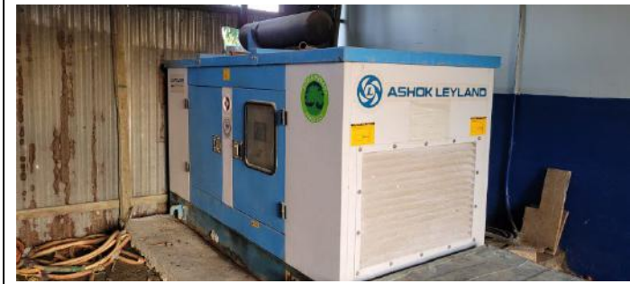
Silent Diesel Generator
