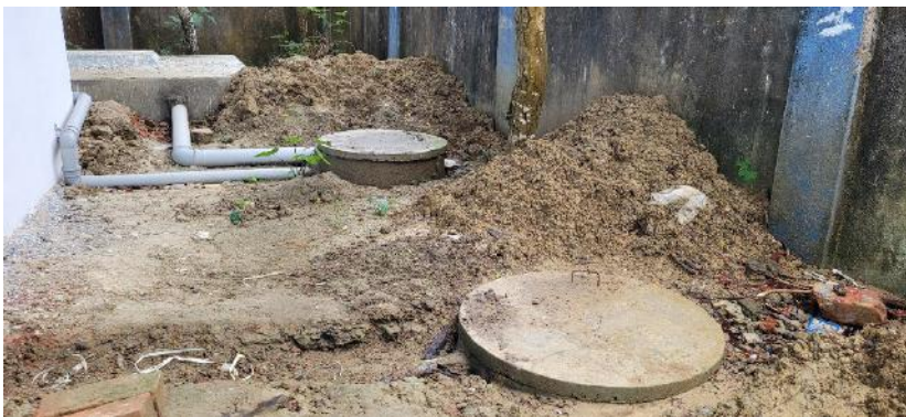
Soak pits for ground water table regeneration
