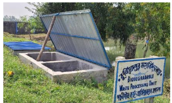
Waste Processing Unit
