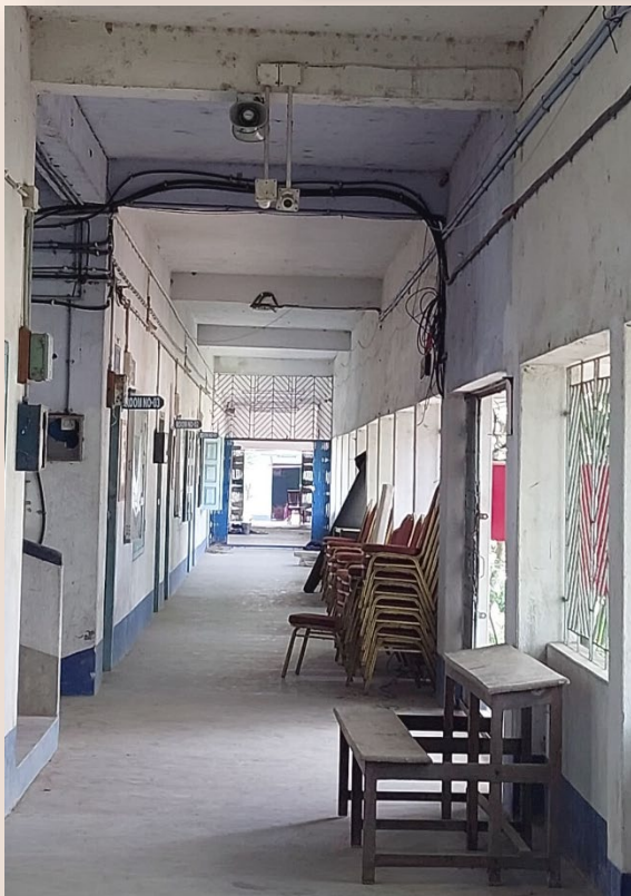
CCTV Cameras & Public Addressing System
